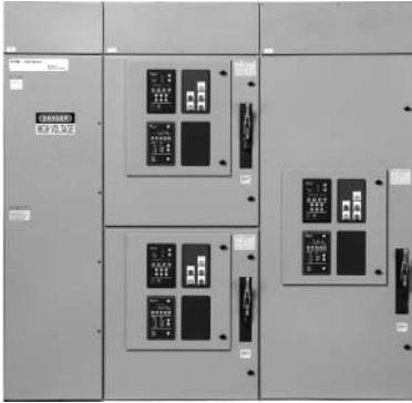
Next Generation AMPGARD Lineup — Front View
