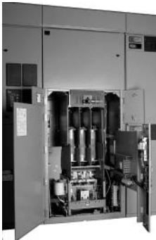
50L7 Vacuum Retrofit
