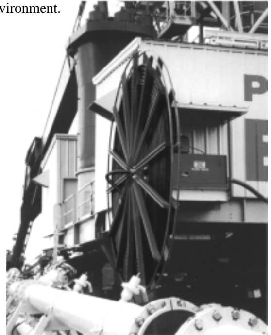
Typical ship loader installation (right)
