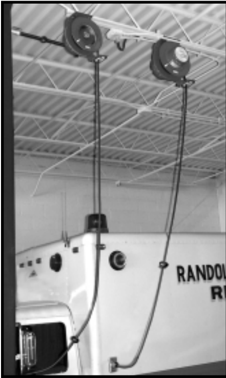
Cable-Master Reels mounted overhead at station provide "off-duty" power to vehicles. Also shown, a Hose-Master to keep air brakes charged. Both can be equipped with sockets which automatically disconnect when engine starts.
